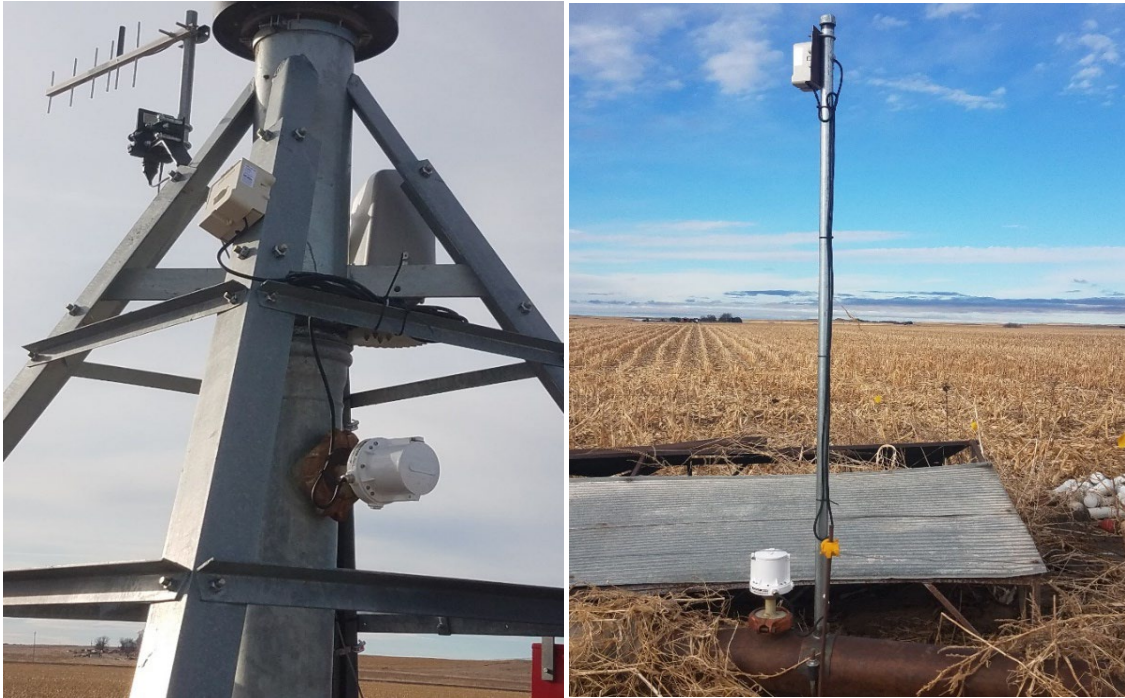
Figure 10. Two different mounting systems for Upper Republican NRD telemetry project.
