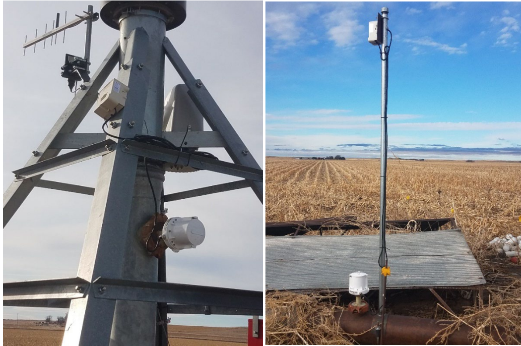
Figure 10. Two different mounting systems for Upper Republican NRD telemetry project.
